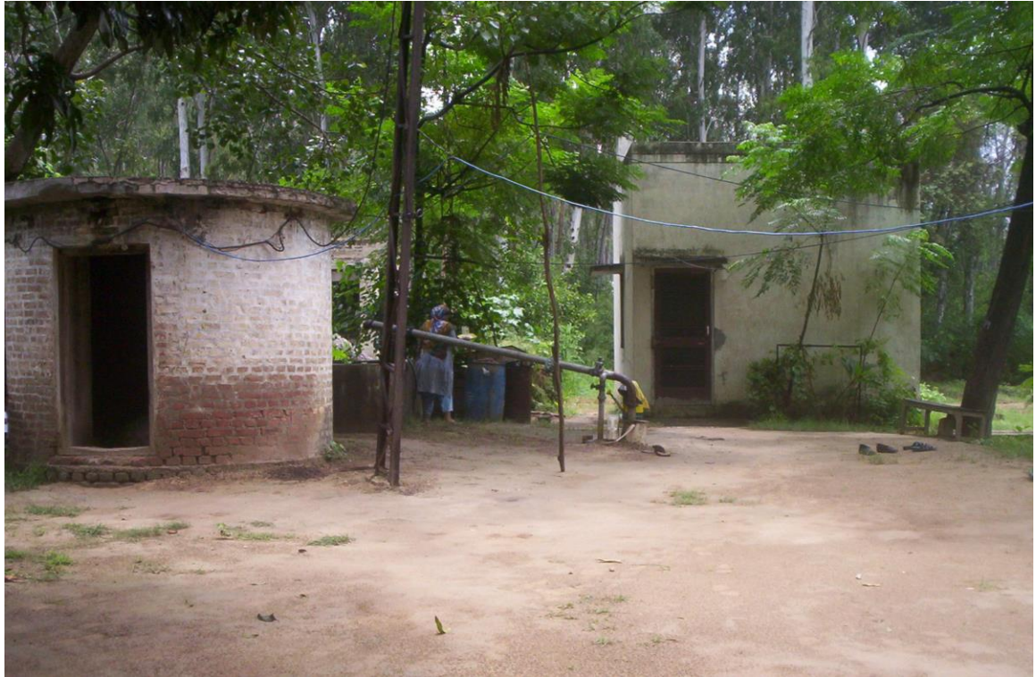
Tubewell pump house in Nursery
